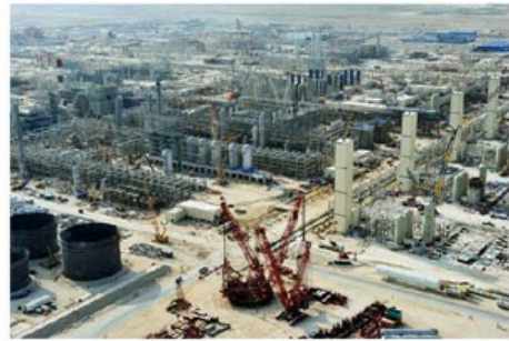
Shell's Pearl Project Gas-to-Liquids Facility in Qatar
